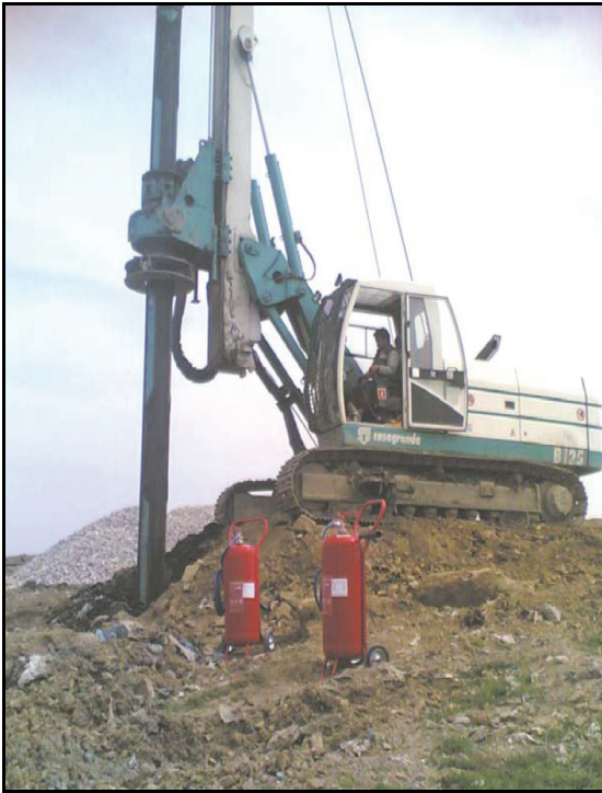
Figure 9. Drilling of a gas well. Because of the methane gas explosion danger, fire extinguishing equipment is kept nearby.
