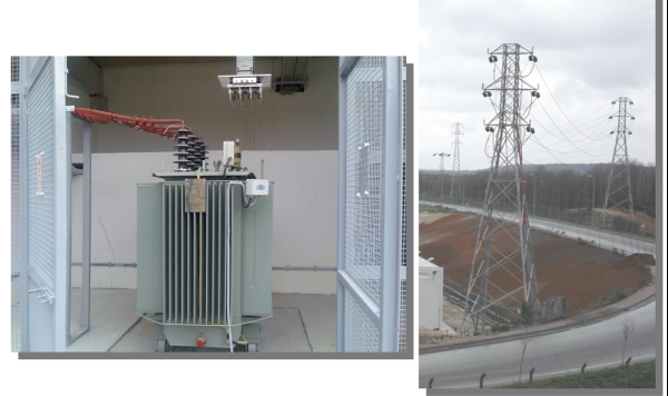
Figure 14. One of the step-up transformers, and the overhead transmission line.
