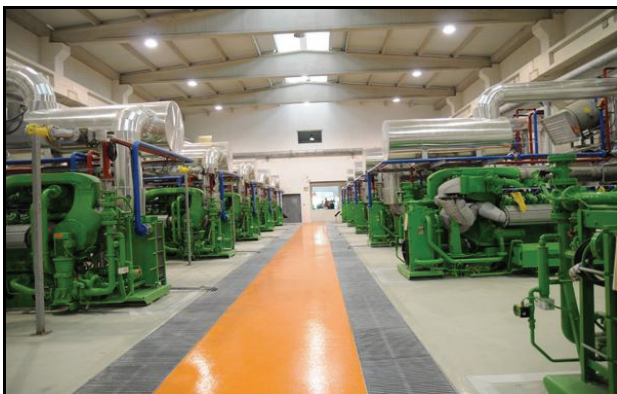
Figure 13. A view from the gen-set hall.
