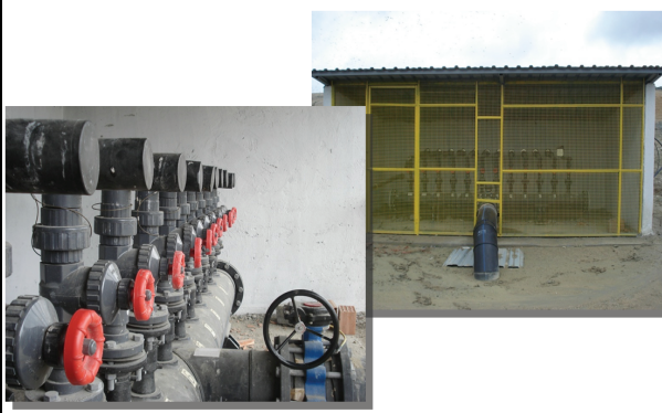
Figure 11. Well pressure regulators and manifold enclosure.
