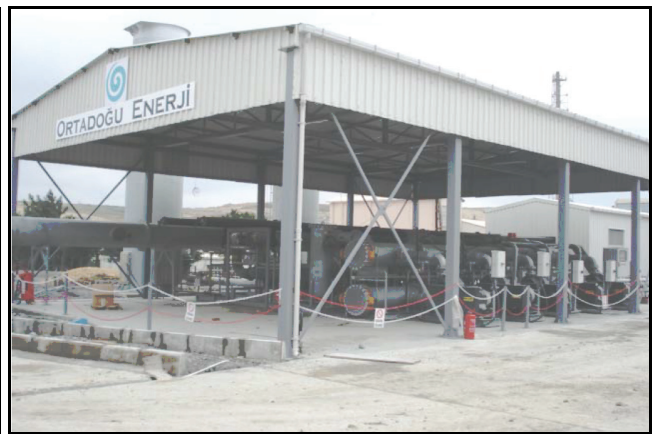
Figure 8. The gas conditioning system and flares.
